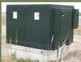
Pad mounted switchgear
