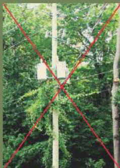
Pole growth contacting electrical equipment & powerlines
