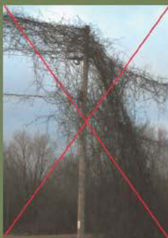
Guy-wire growth contacting electrical equipment & powerlines
