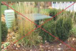
Obstruction around a transformer
