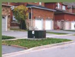
Pad mounted transformer
