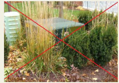
Obstruction around a transformer
