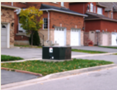
Pad mounted transformer
