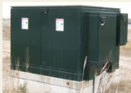
Pad mounted switchgear
