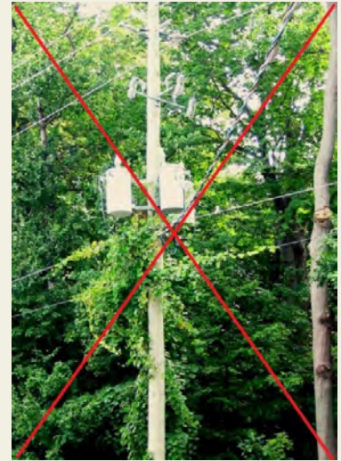
Pole growth contacting electrical equipment & powerlines
