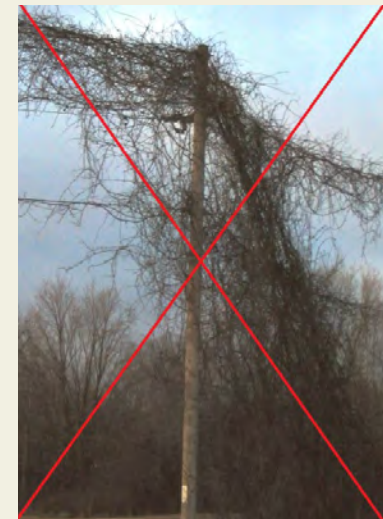
Guy-wire growth contacting electrical equipment & powerlines
